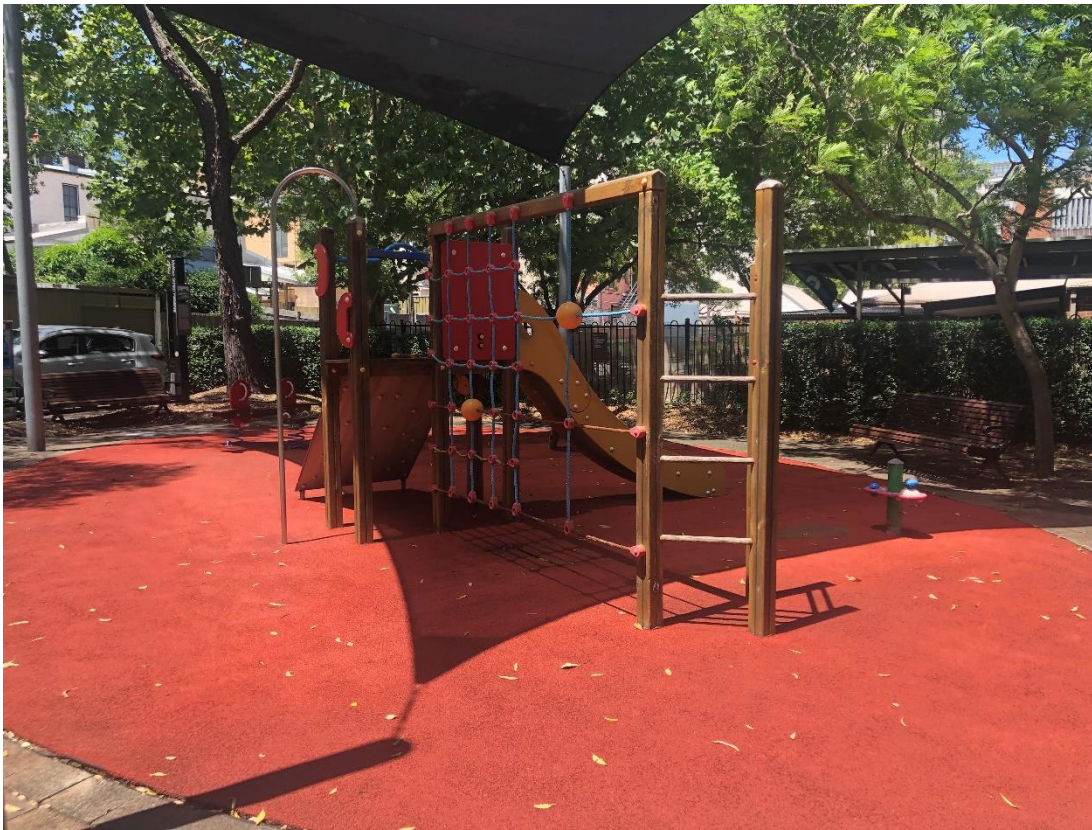
Existing playground in the reserve – play equipment is at the end of its lifecycle; soft-fall is worn and separating from edges. Playground is well shaded from the existing trees and shade structure.
