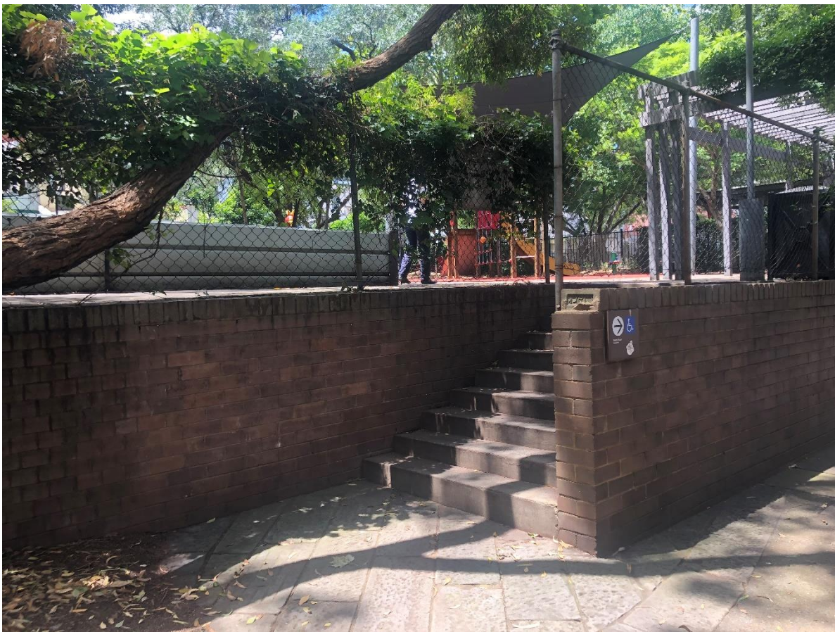
Existing stairs from Wattle Lane (to be retained). Movement and cracking of brick retaining wall.
