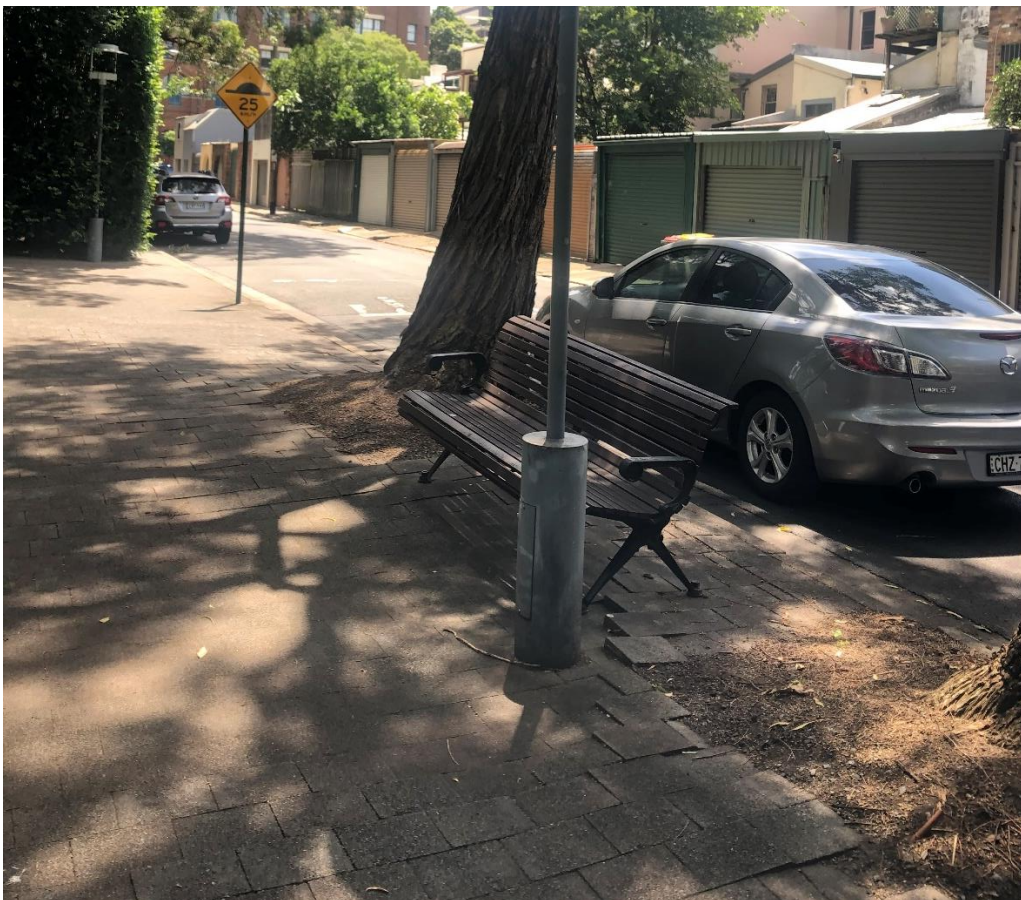
Looking north along McKee Street. Uneven paving along the footpath due to tree roots.
